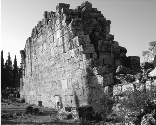
Fig.1 Baths-Church. The east wall leans as a result of earthquakes.
